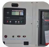
Control Panel & MCB
